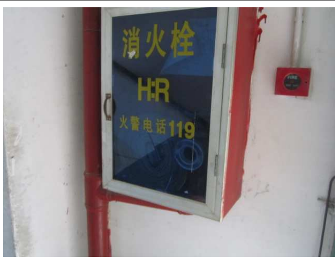
Fire hose & fire alarm
